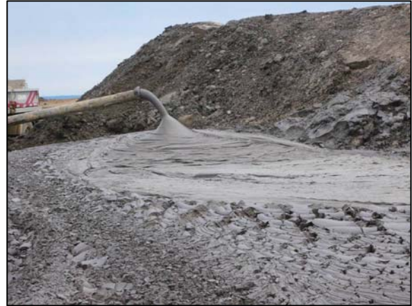
Figure 7. Paste discharge and illustration of deposition angle. Note surface cracking of deposited paste
