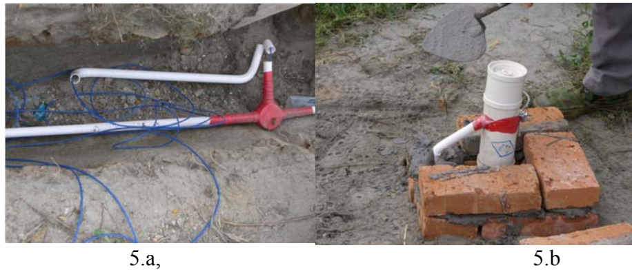
Figure 5. a) Schematic diagram of monitoring system; 5.b) installation and protection of the sensors and fiber optic cable.
