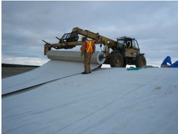
Figure 3. Deployment of the GCL. One foot overlap being done. Polypropylene side of the GCL facing down.
