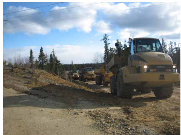
Figure 2. Hazco's truck fleet carrying the clay from a nearby clay source available on site being transported as a cover soil over the geosynthetic clay liner.
